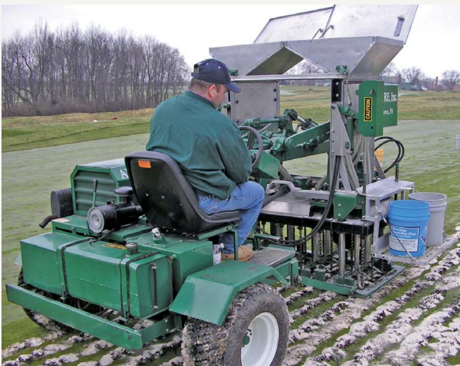
Among the renovation practices used at Oakmont is 'drill-n-fill', where 12-inch (30cm) holes are drilled down to within inches of the sub-surface drainage lines to promote deeper root growth and superior drainage
